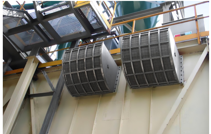
Explosion venting of a chip bunker using the Q-Box to protect the surrounding infrastructure.
